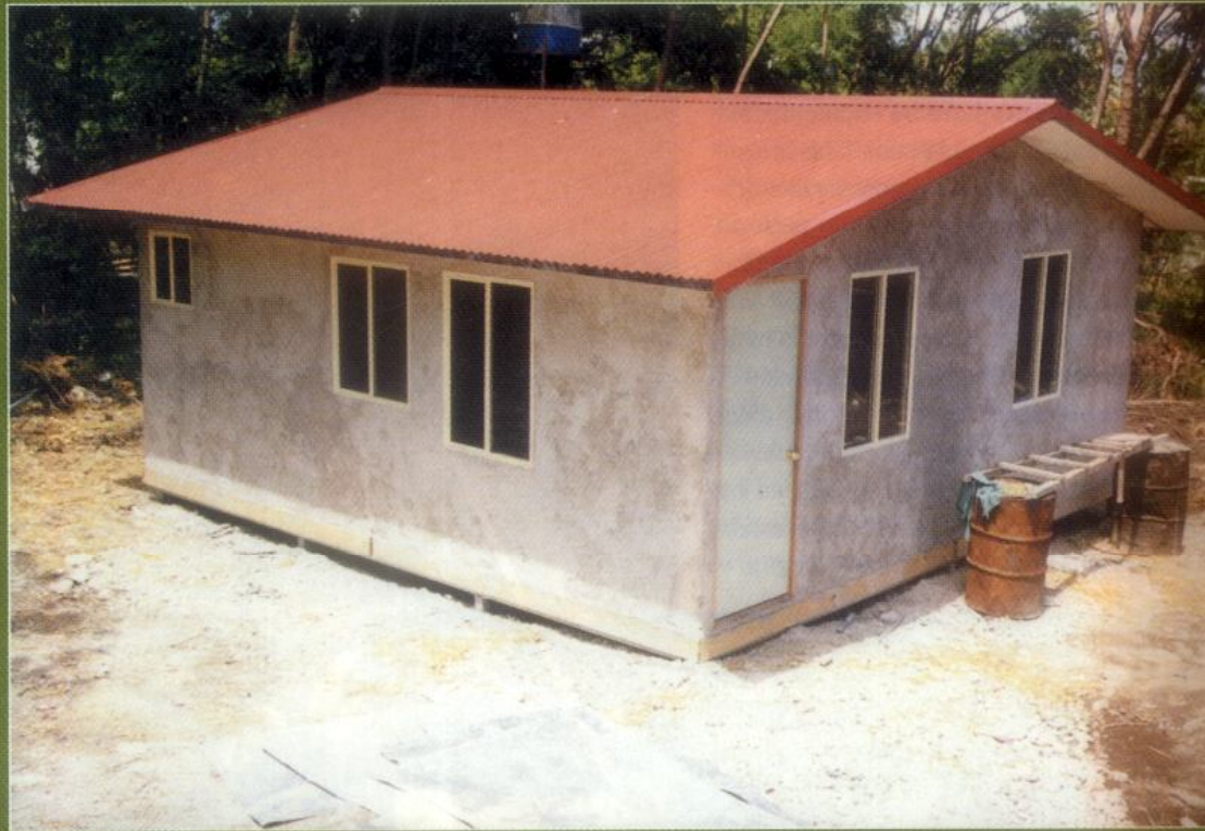
This prefabricated house was built by Ortech Industries in less than four days using a combination of Australian and East Timorese tradespeople.
